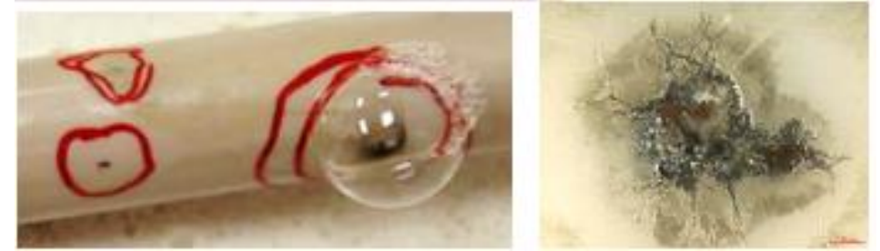
Damaged coolant lines
