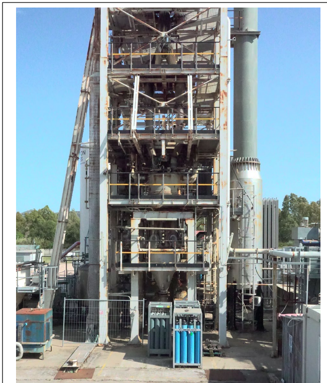
Figure 1. Photograph of a demonstration scale updraft moving bed gasifier at Sotacarbo SpA. The reactor has an inner diameter of 1.3 m and is capable of gasifying 10,000 tons per year of solid waste carbon (e.g. coal, biomass and/or plastic). Photo courtesy of Hamilton Maurer International.
